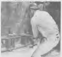
EACH OF THE 24 nuts was tightened to a pressure of approximately 1000 pounds.
